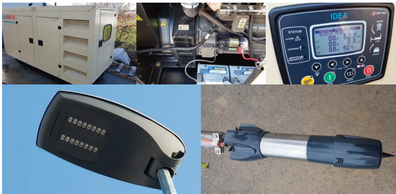
Fig. 12. The electric generator, lighting system and lightning protection
