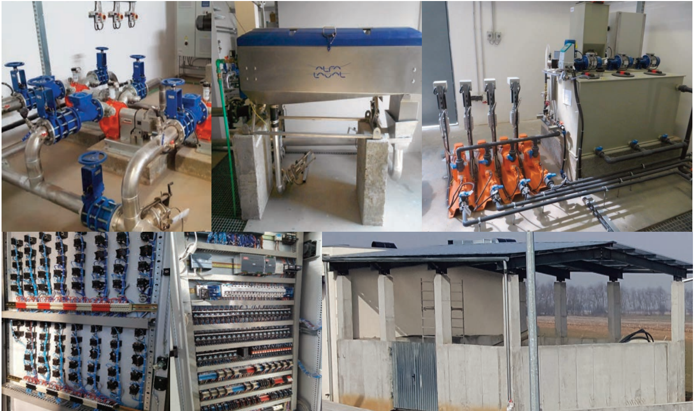
Fig. 8. Sludge treatment stage
